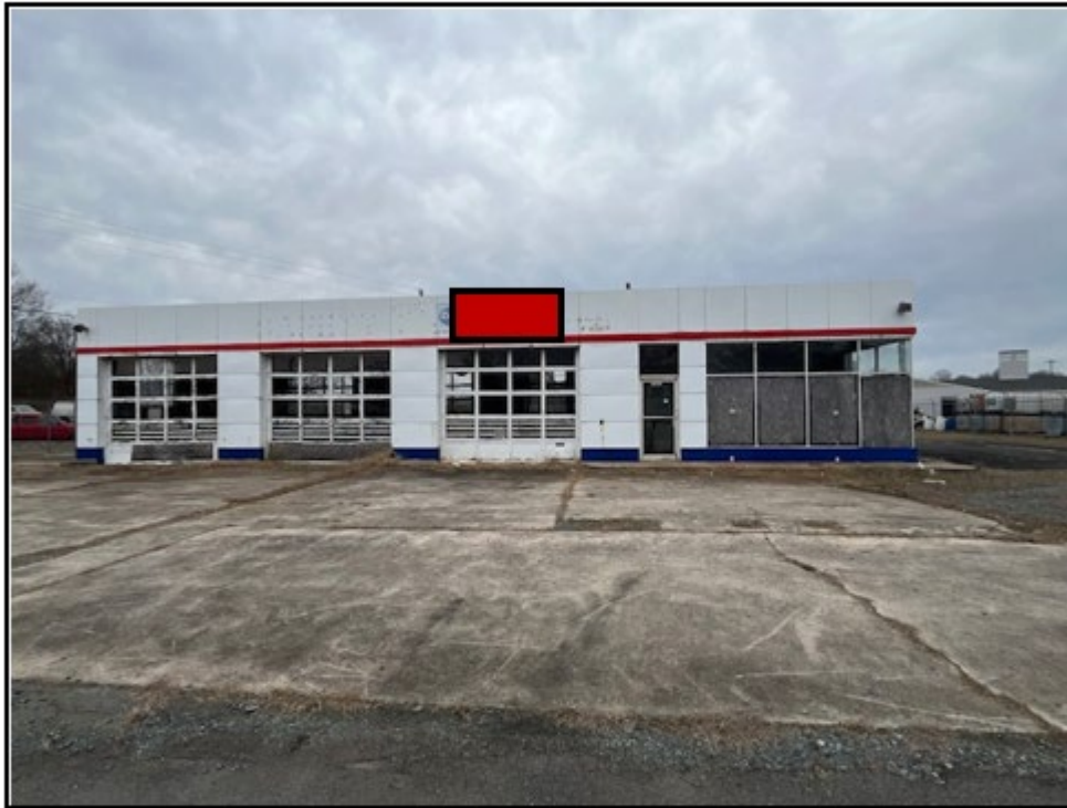
Subject property: 6349 W. Marshville Hwy. (old Cooper Tire/Amoco site) Façade size: 1,008 square feet Depicted sign size: 32 square feet (3 percent of façade size)
